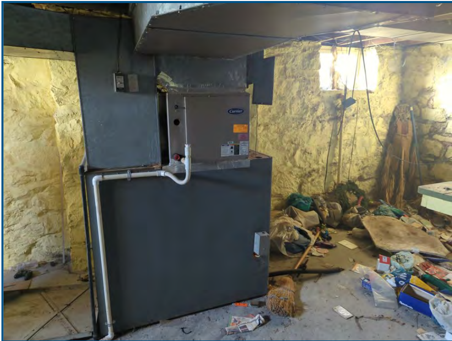
Photograph # 6 View of the furnace in the basement.
