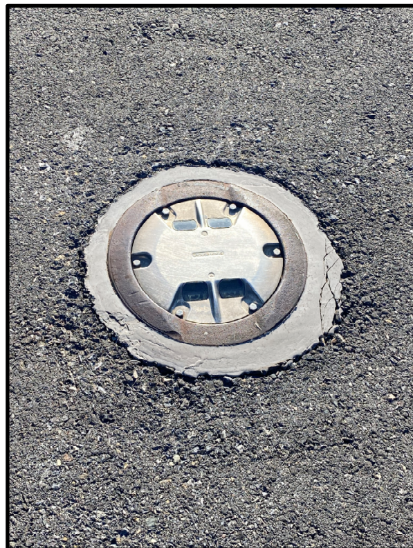
Figure 5.1 – Existing Light Fixtures
