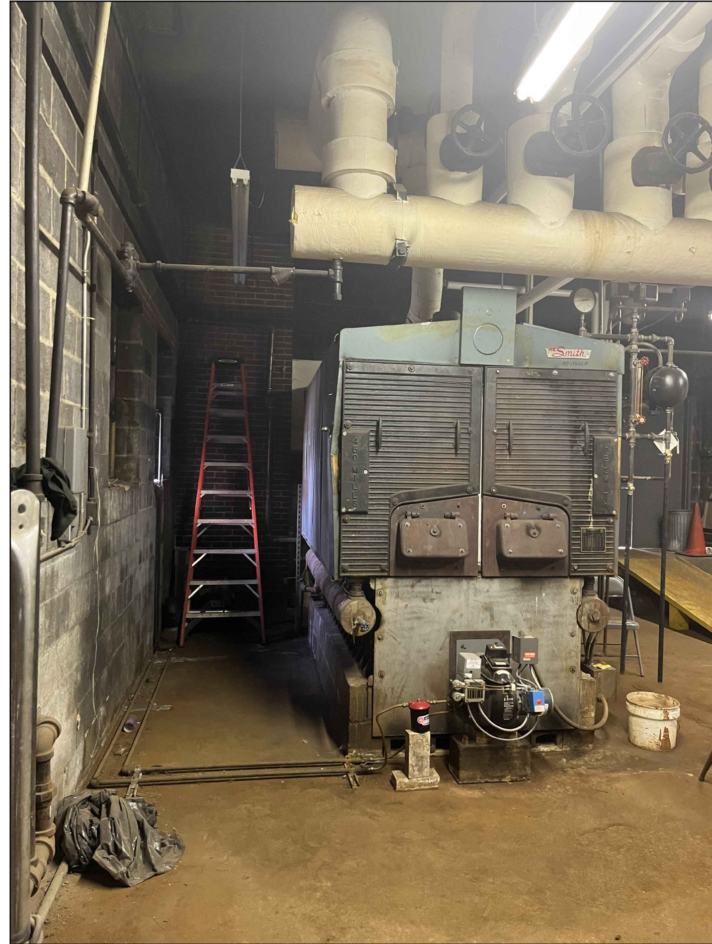
EXHIBIT #2: H.W. BOILER
