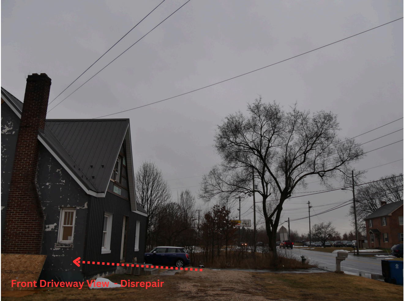
Front Driveway View - Disrepair
