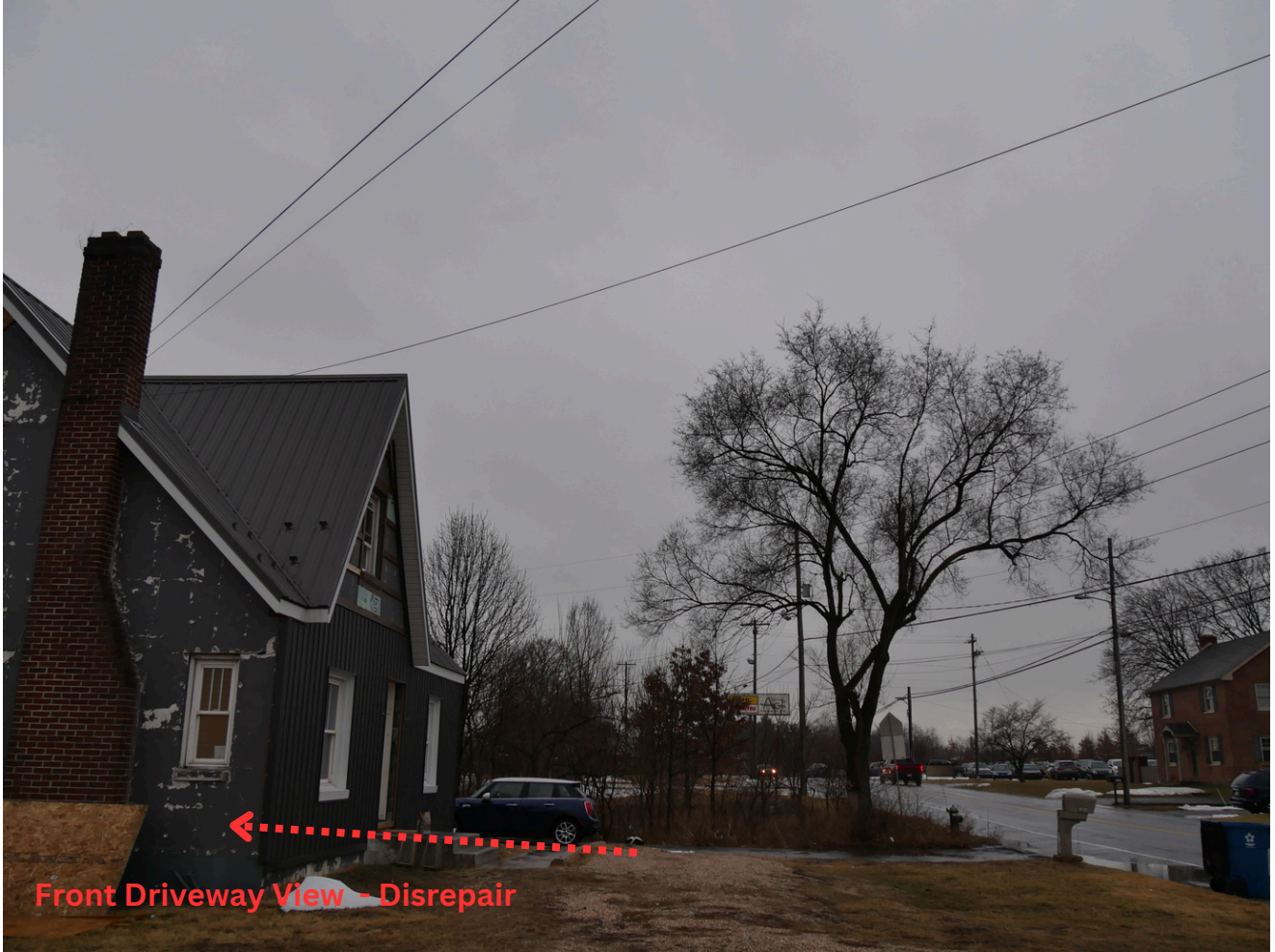
Front Driveway View - Disrepair
