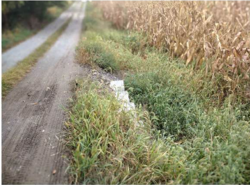
Photograph 23 – Looking northwest at fill activity and drainpipe installation in the proposed access/utility easement.
