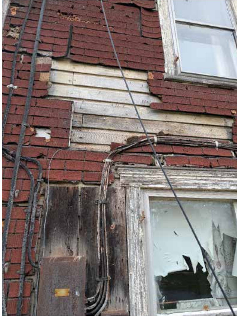
Photo 8: Window trim detail and additional siding condition photo; infrastructure condition
