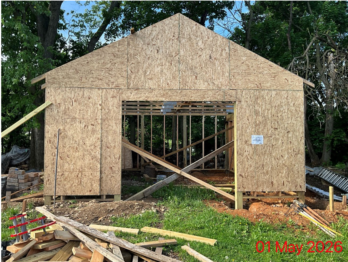
Photo 4: View of Construction at time of stop work (source: SR2026-0113); facing south
