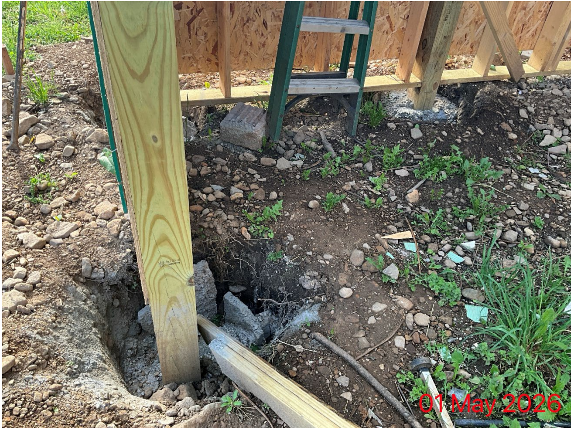
Photo 6: View of Construction at time of stop work (source: SR2026-0113), detail of footer
