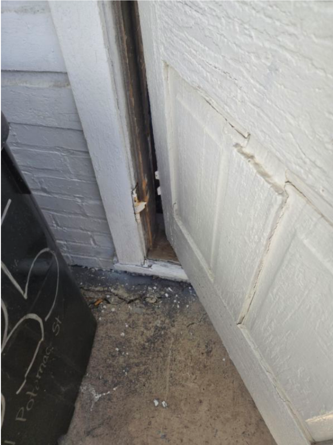
20. Exterior door leading to basement damaged (hinge broken)
