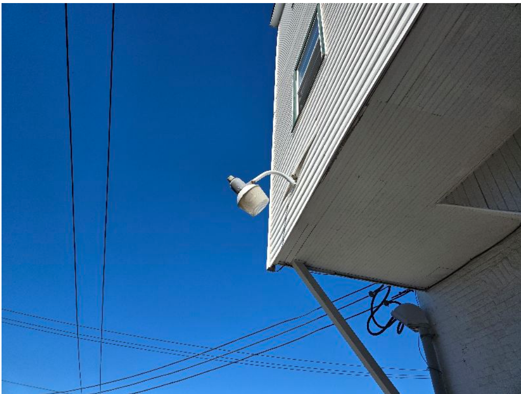
19. Damaged light fixture needs to be removed/replaced (rear addition)
