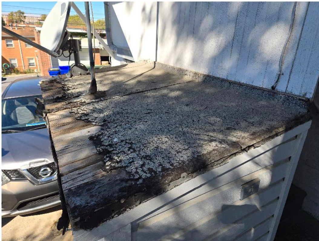
17. Deteriorated roof (basement entry stairs)
