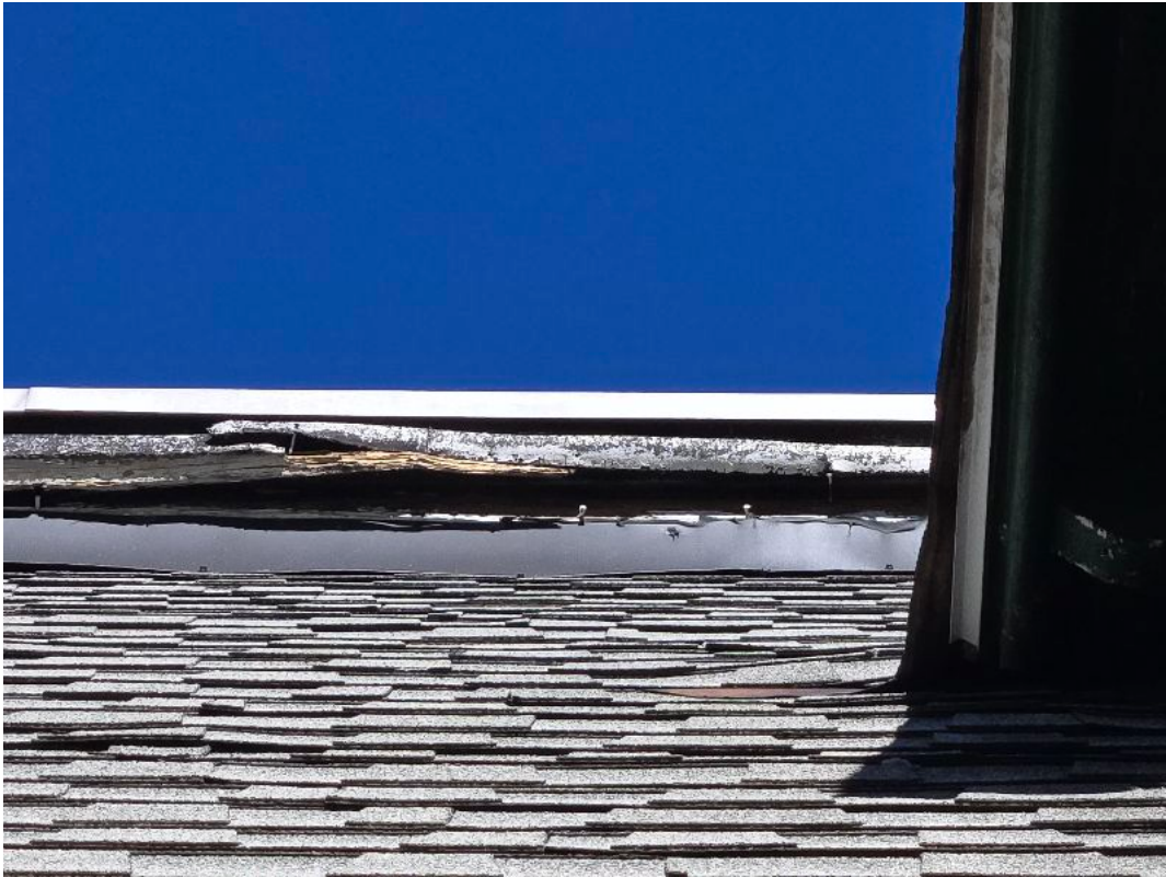
12. Damaged ridge line flashing (south side)
