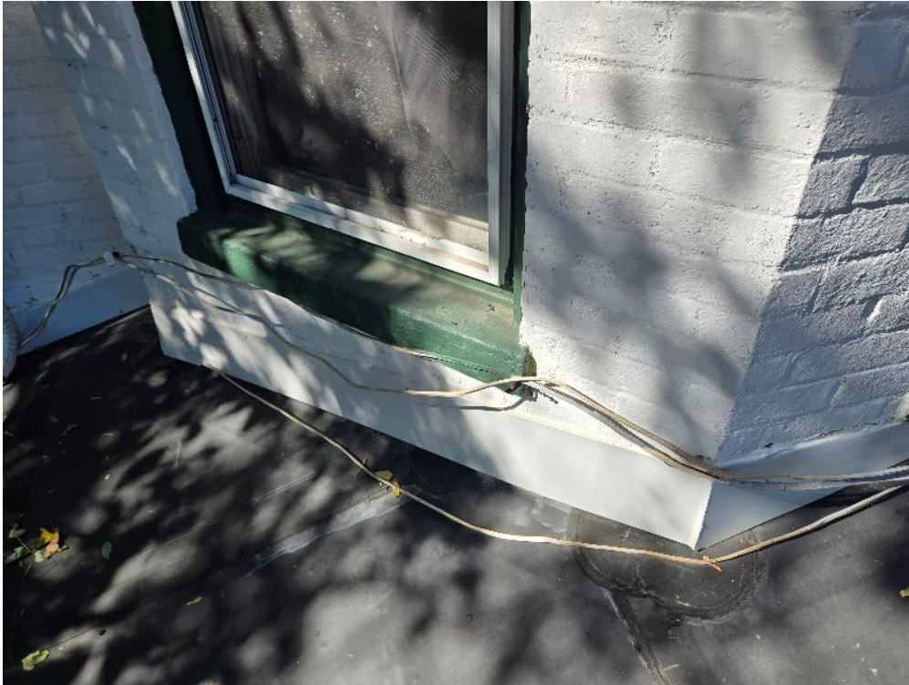
18. Wiring not UV rated, needs to be replaced (front, 2nd story)
