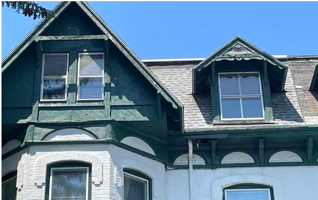
1. Peeling paint on front facade
