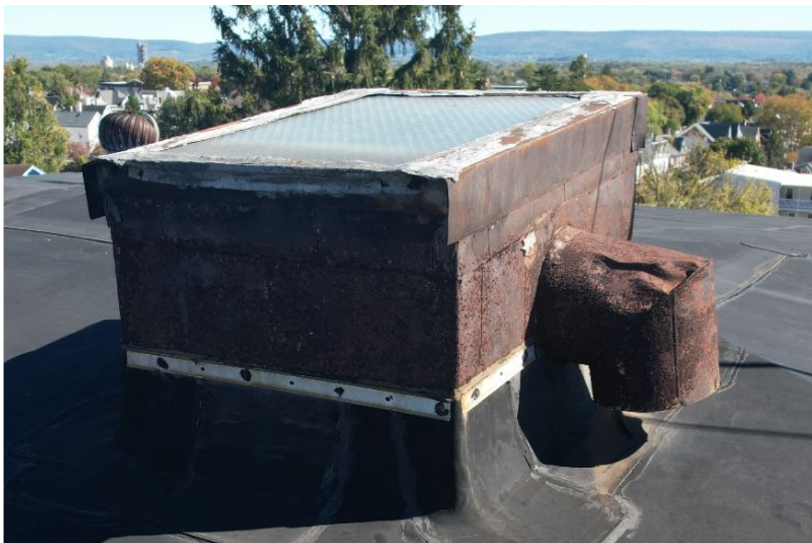
7. Skylight housing corroded
