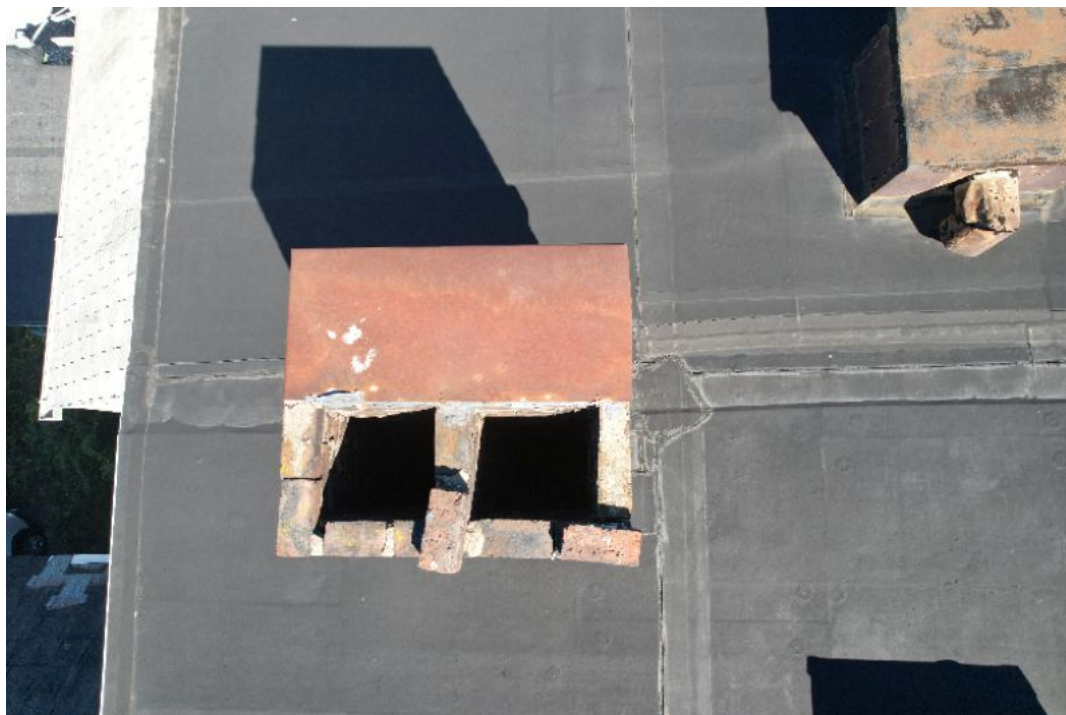
5. Chimney cap needed
