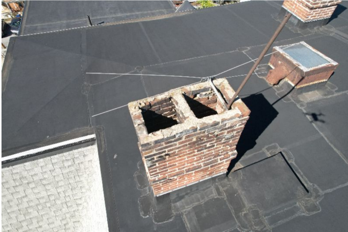
6. Chimney cap needed
