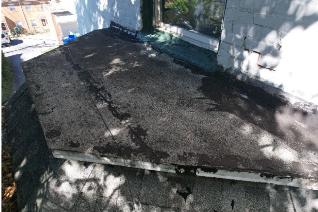
16. Deteriorated roof (south side bay window)
