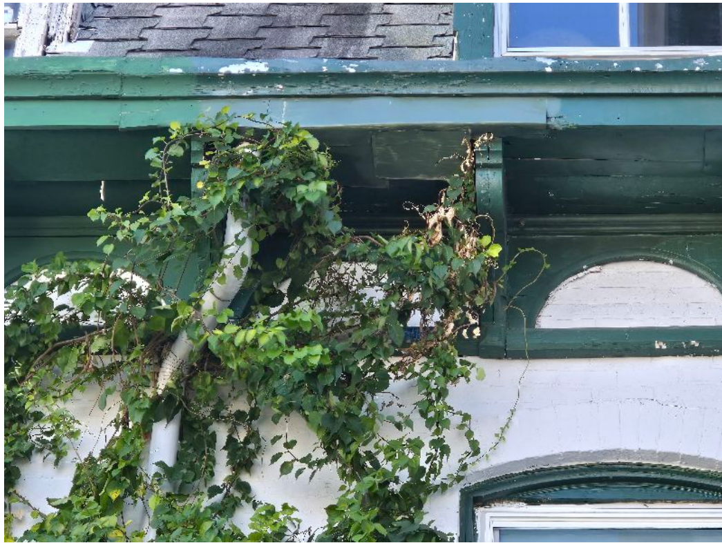
4. Damaged soffit (rear)
