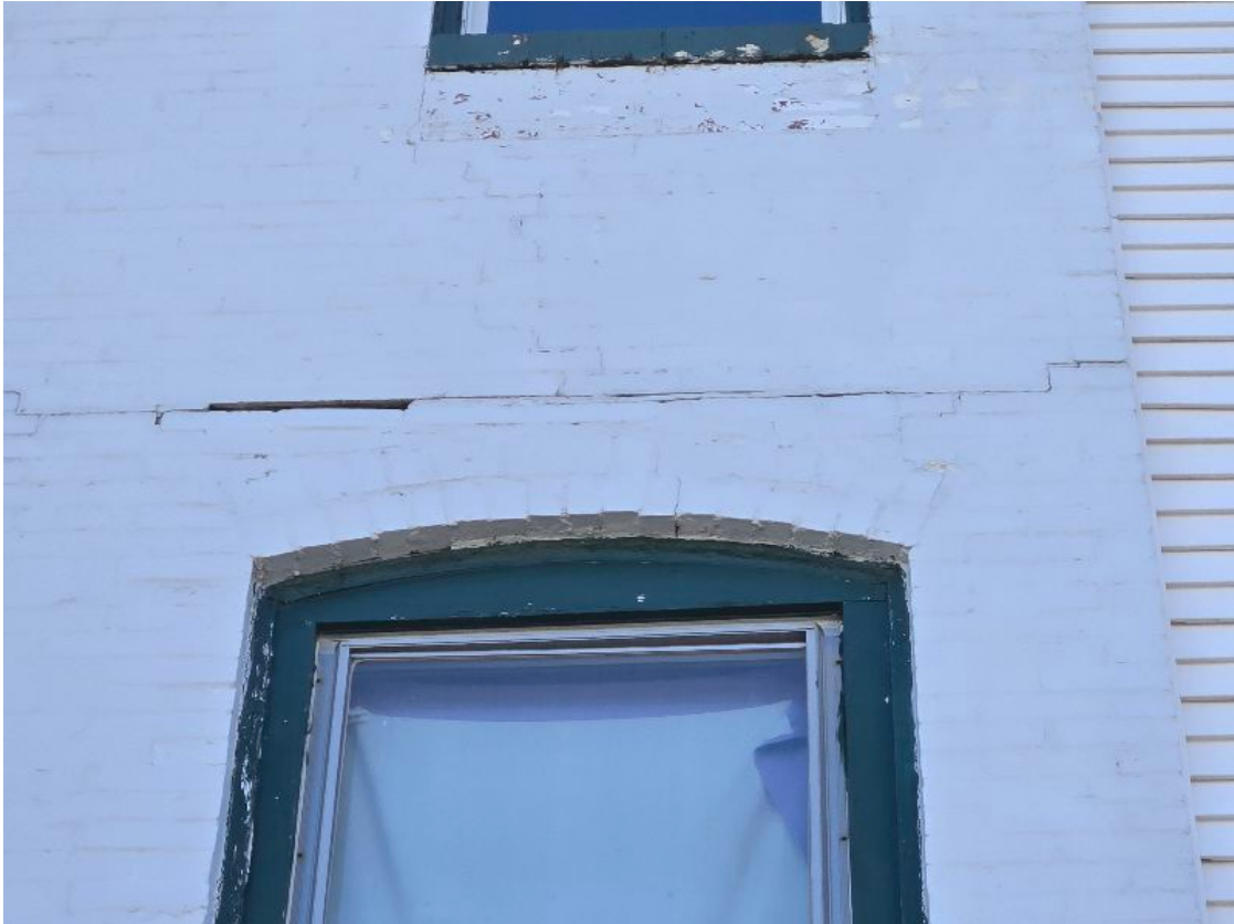
9. Masonry Cracks (rear of building)
