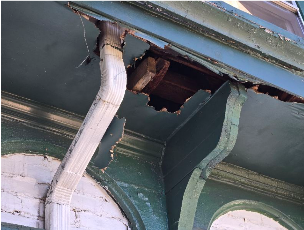
3. Damaged soffit (front)
