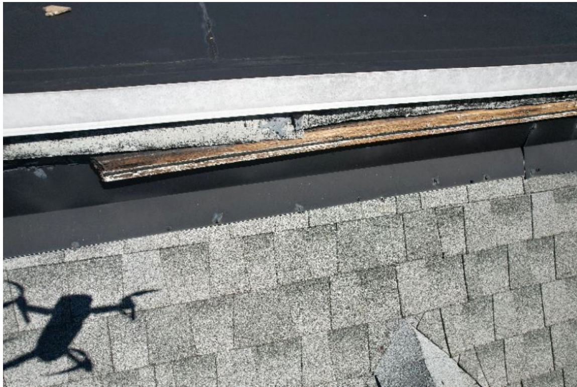
10. Damaged ridgeline flashing (south side)
