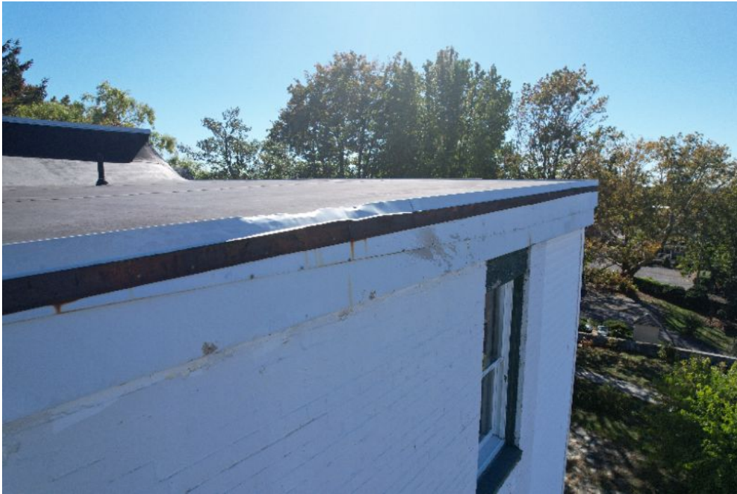
14. Damaged flashing (rear)
