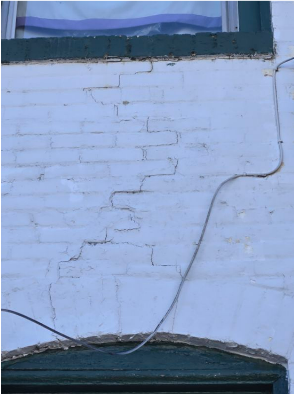
8. Masonry Crack (rear of building)
