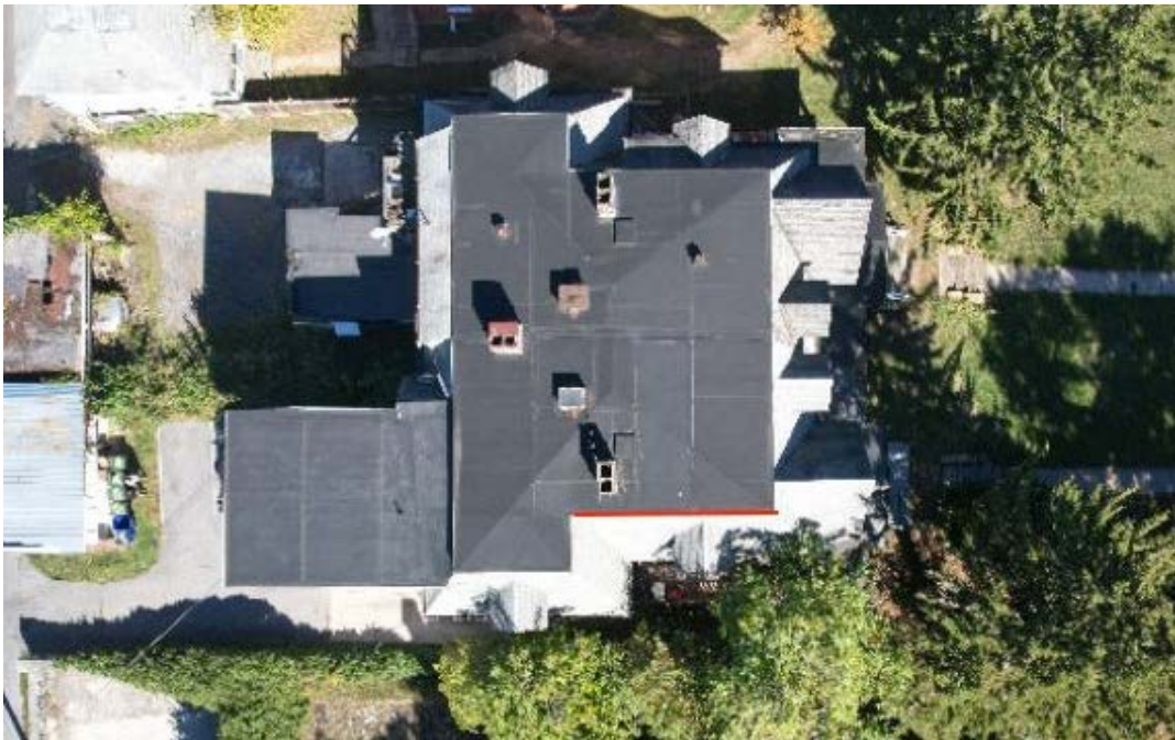
13. Area of damaged ridge line flashing (appx 40 linear feet)
