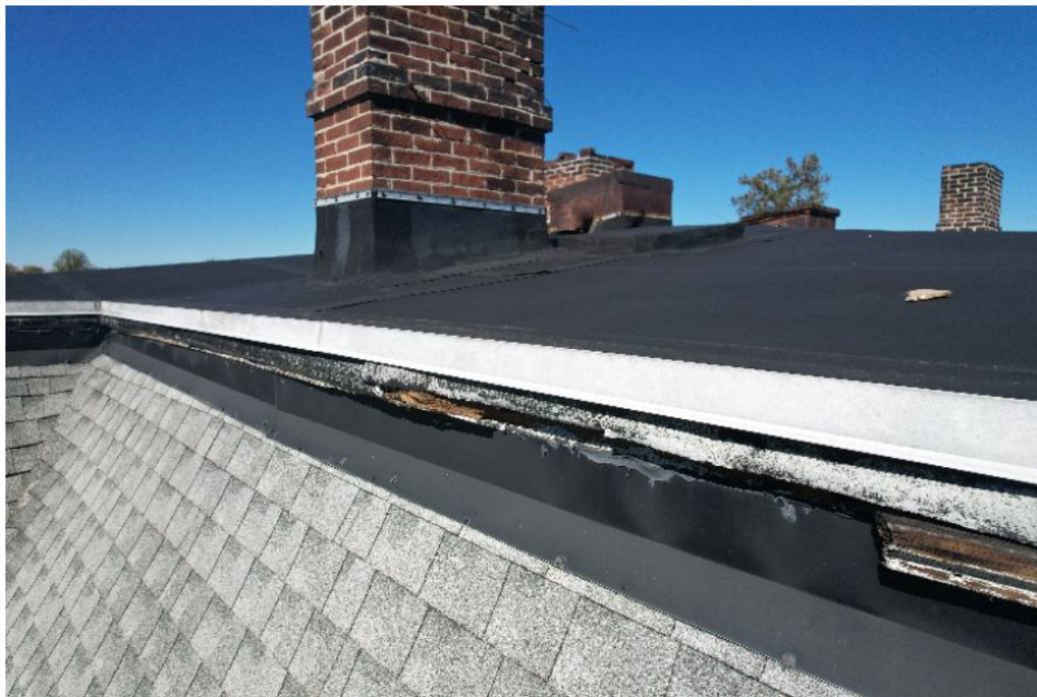
11. Damaged ridgeline flashing (south side)
