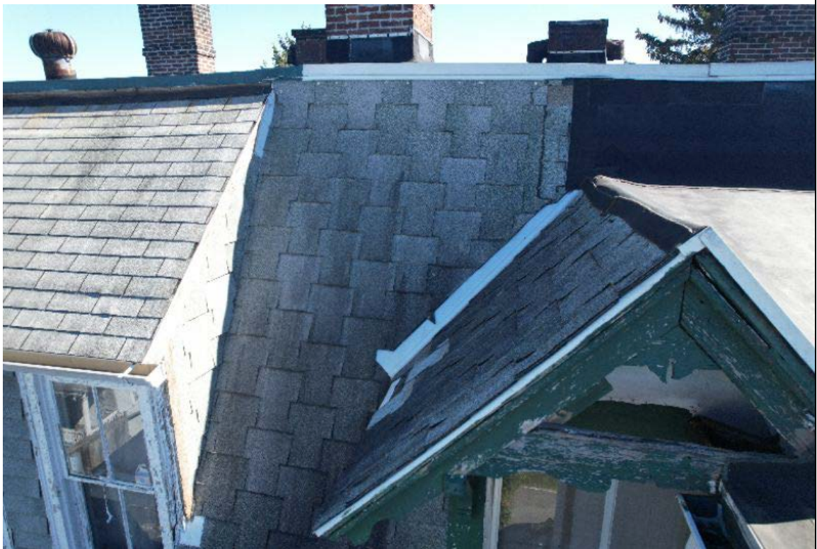
2. Peeling paint rear dormer
