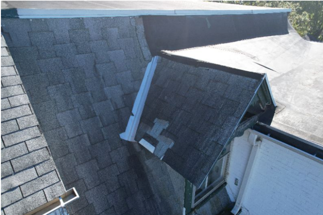
15. Missing shingles (west side dormer)
