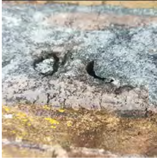
1-1, Cracker Mortar at chimney crown
