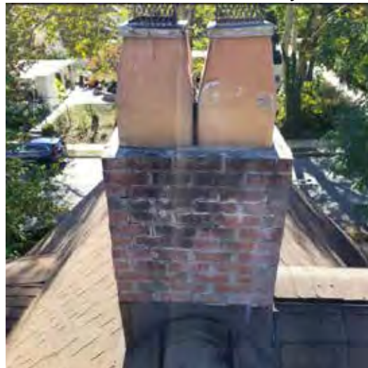
1-2, chimney showing condition of mortar and crown
