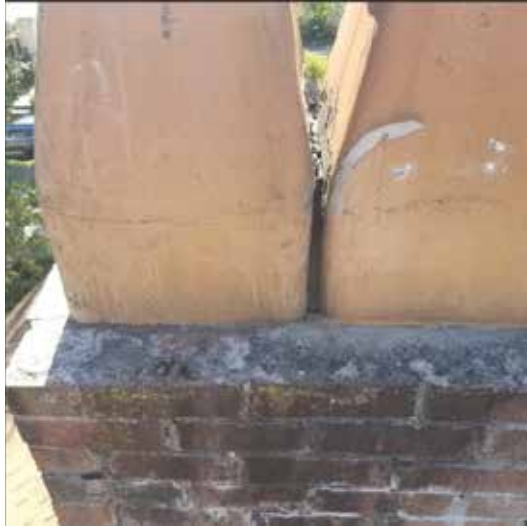
1-4, Chimney thimble condition showing cracks
