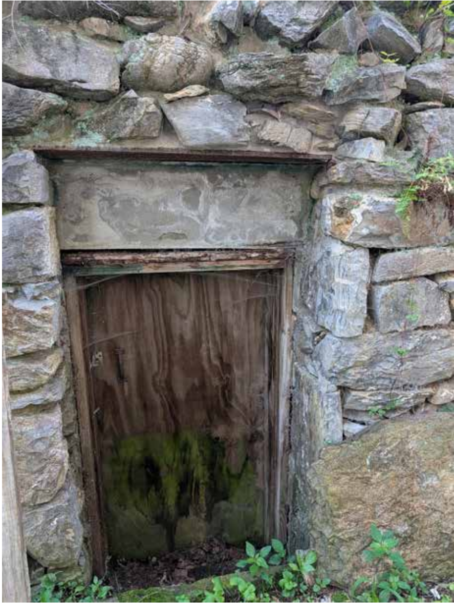
5_well pump house, adjacent to east side of house
