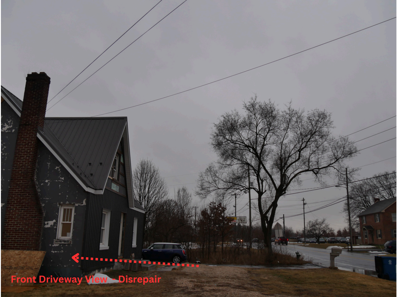
Front Driveway View - Disrepair
