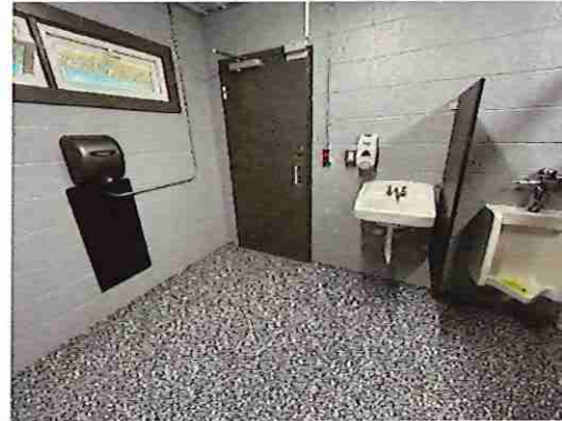
Pavilion #2 Men's Toilet Room Sink
