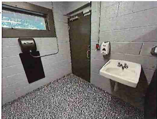
Pavilion #4 Men's Toilet Room Sink
