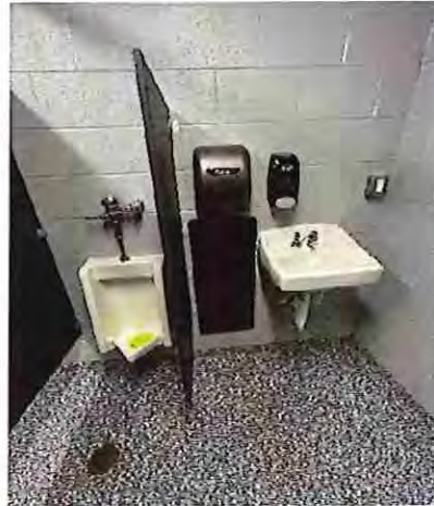
Little League Right Toilet Room Sink
