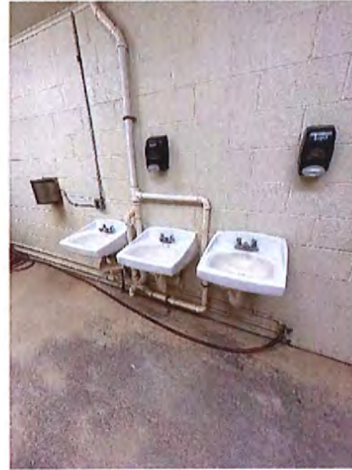
Men's Toilet Room Sinks
