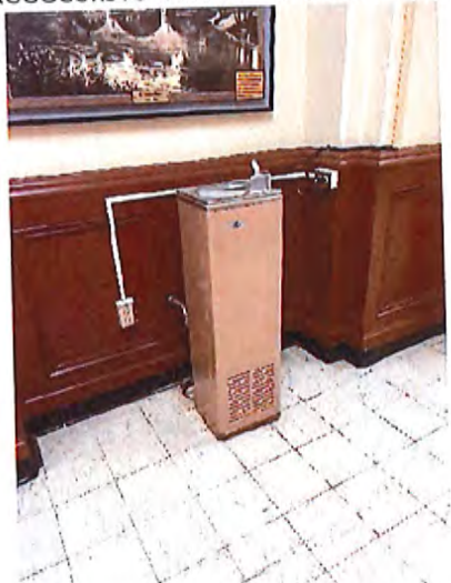
1 st Floor Drinking Fountain
