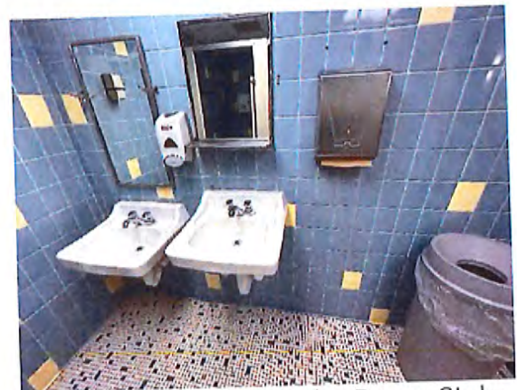
3rd Floor Women's Toilet Room Sinks
