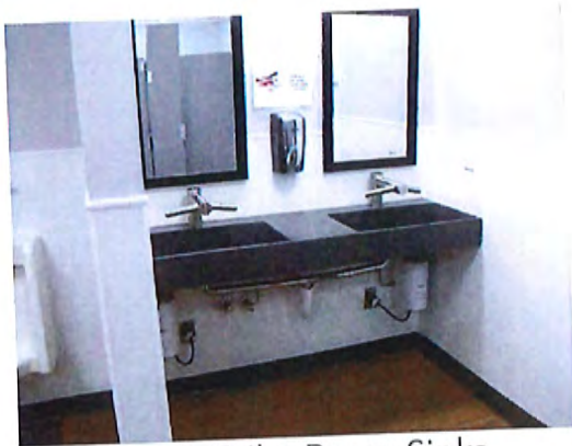
Men's Toilet Room Sinks
