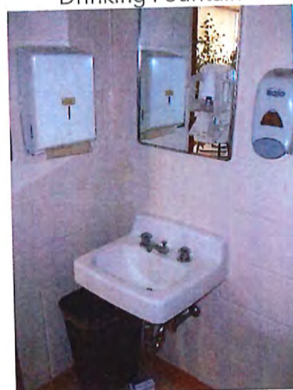
Men's Toilet Room Sink
