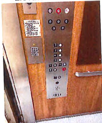
Elevator Control Panel
