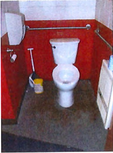
Toilet Room Accessible Water Closet
