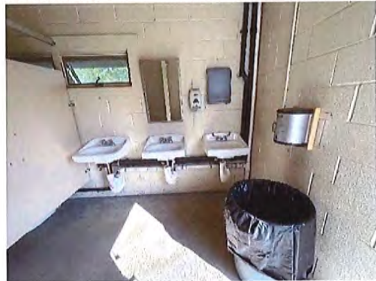
Men's Toilet Room Sinks
