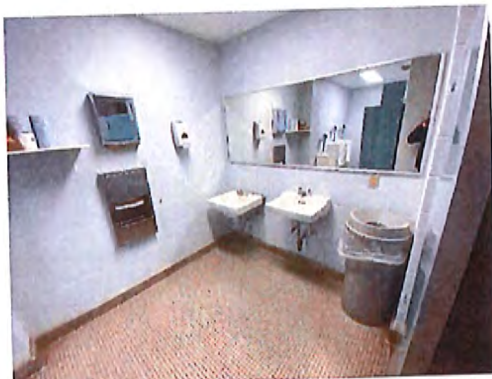
2 nd Floor Men's Toilet Room Sinks
