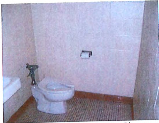
Men's Toilet Room Water Closet
