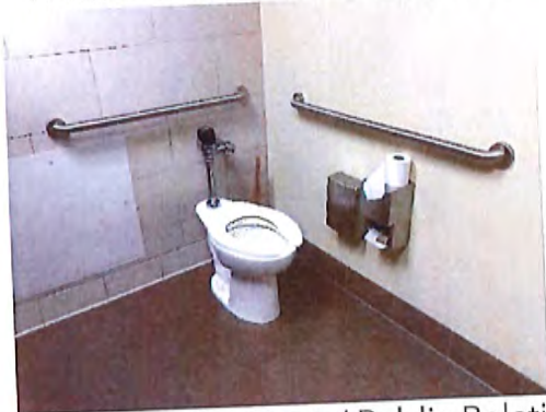
Business Development / Public Relations Women's Toilet Room Water Closet
