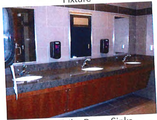
Men's Toilet Room Sinks
