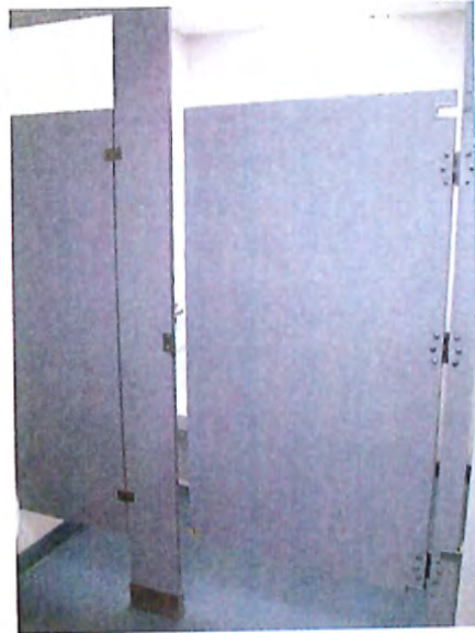
Toilet Room Stall Fixture
