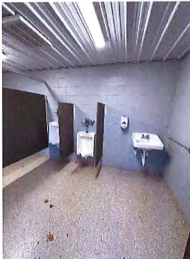
Men's Toilet Room Sink
