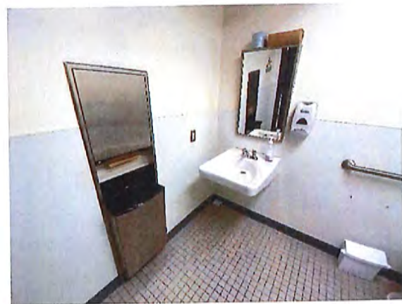
Women's Toilet Room Sink
