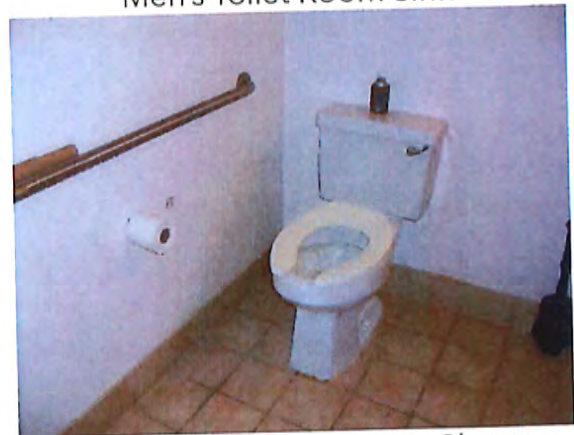
Men's Toilet Room Water Closet
