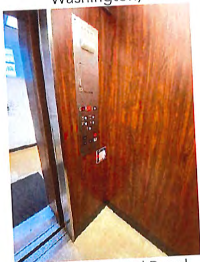
Elevator Control Panel
