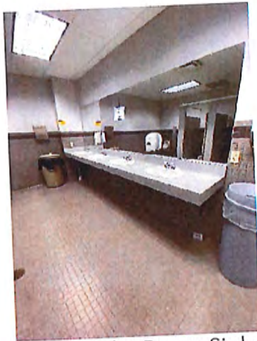
Men's Toilet Room Sinks
