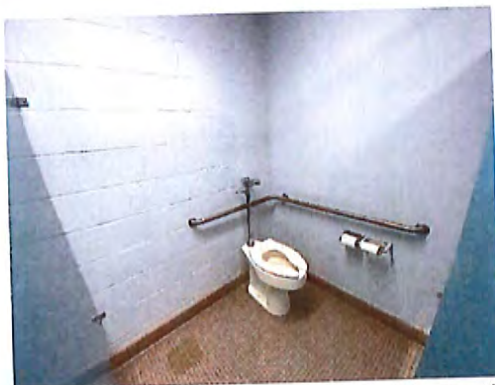
2 nd Floor Men's Toilet Room Accessible Water Closet / Stall
