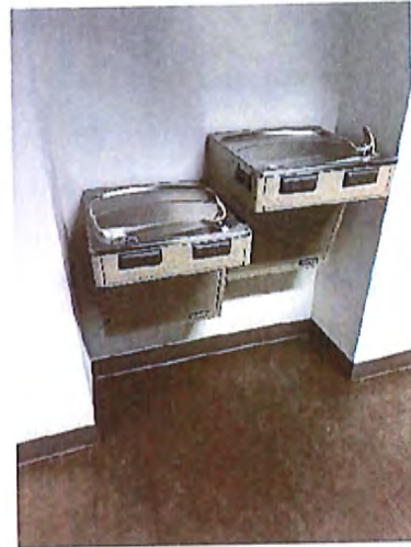
2 nd Floor Drinking Fountains
