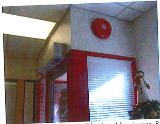
Main Entrance Door Closing Hardware & Fire Alarm
