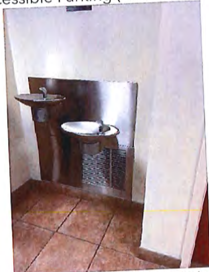
1st Floor Drinking Fountain
