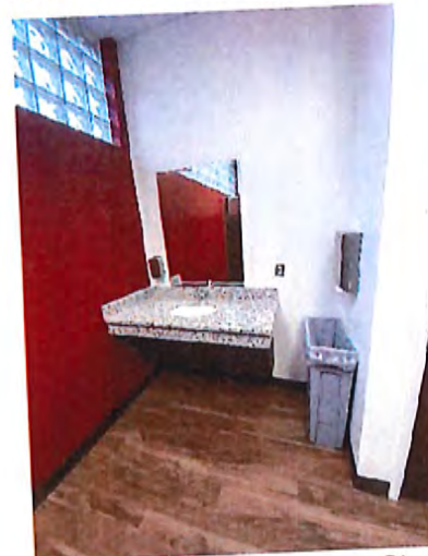
Women's Toilet Room Sink
