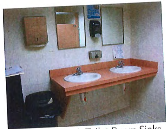
(Right) Women's Toilet Room Sinks
