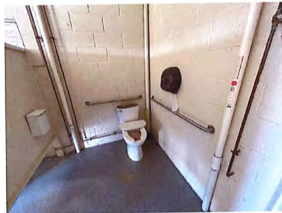
Women's Toilet Room Accessible Water
