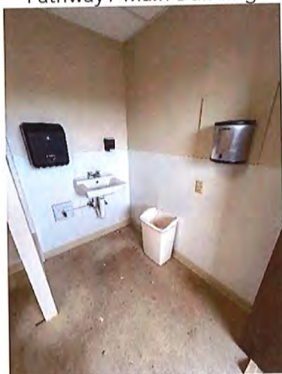
Men's Toilet Room Sink
