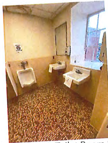
3rd Floor Men's Toilet Room Sinks
