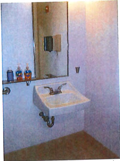
Women's Toilet Room Sink
