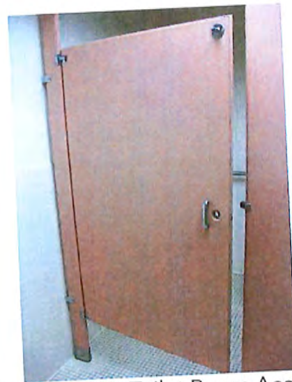
(Right) Women's Toilet Room Accessible Stall Door
