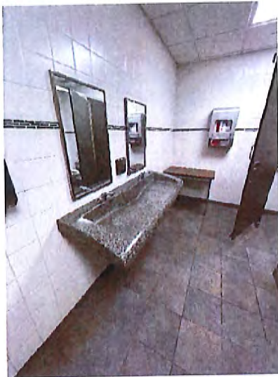
2 nd Floor Women's Toilet Room Sink
