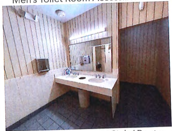
Women's Toilet Room Sink / Route
