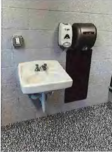
Pavilion #3 Men's Toilet Room Sink
