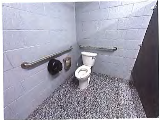
Southern Pavilion Left/North Toilet Room Accessible Water Closet / Stall
