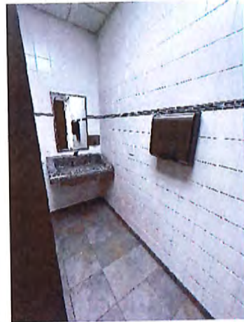
1st Floor Women's Toilet Room Sink
