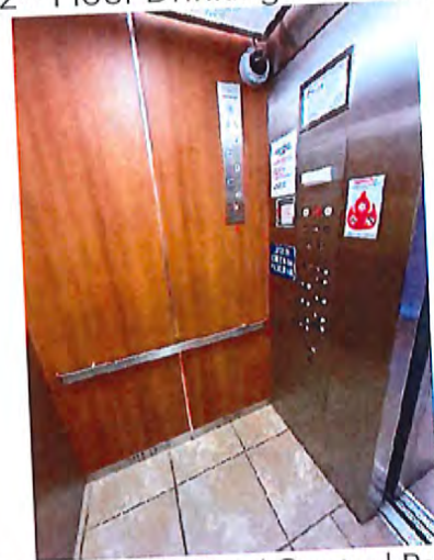
Elevator Interior / Control Panel
