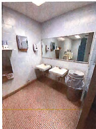
3 rd Floor Men's Toilet Room Sinks
