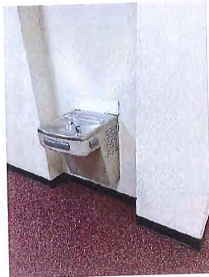
3 rd Floor Drinking Fountain
