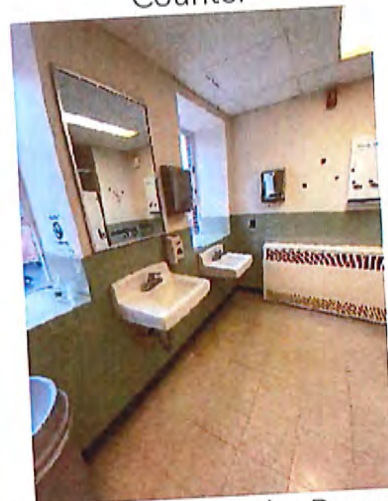
3rd Floor Women's Toilet Room Sinks
