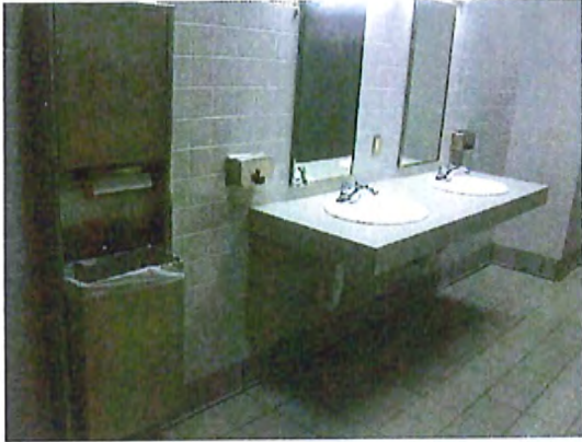
Men's Toilet Room Sinks
