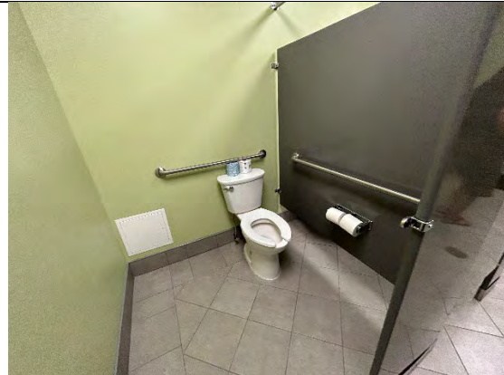
Front Men's Toilet Accessible Stall
