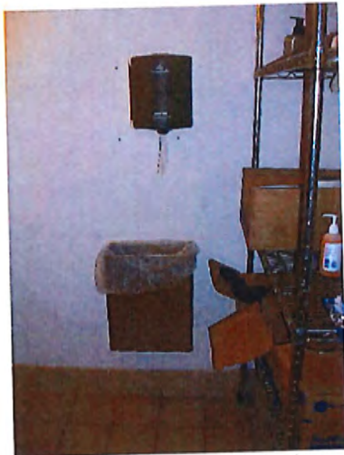
Men's Toilet Room Hand Dryer
