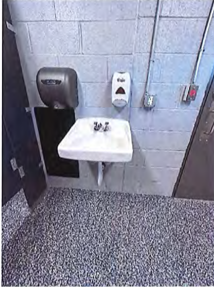
Upper Pavilion - Women's Toilet Room Sink
