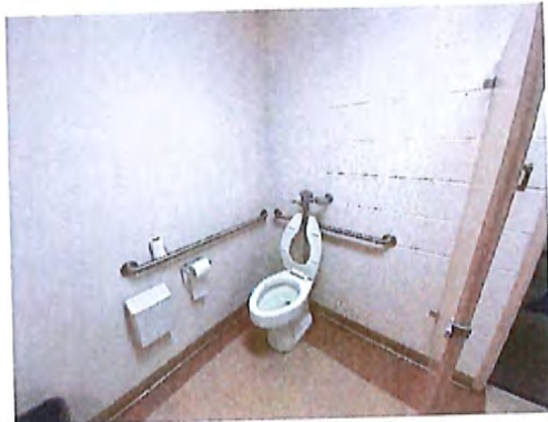
2 nd Floor Women's Toilet Room Accessible Water Closet / Stall
