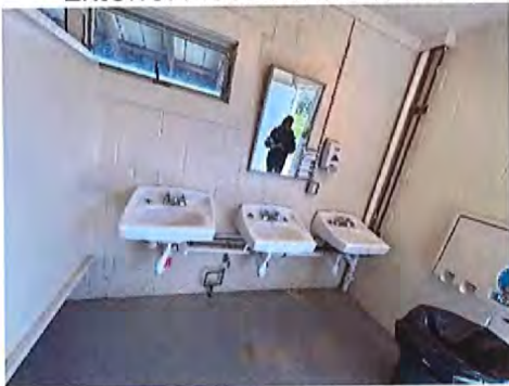
Men's Toilet Room Sinks
