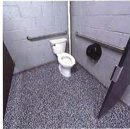
Upper Pavilion - Men's Toilet Room Accessible Water Closet / Stall
