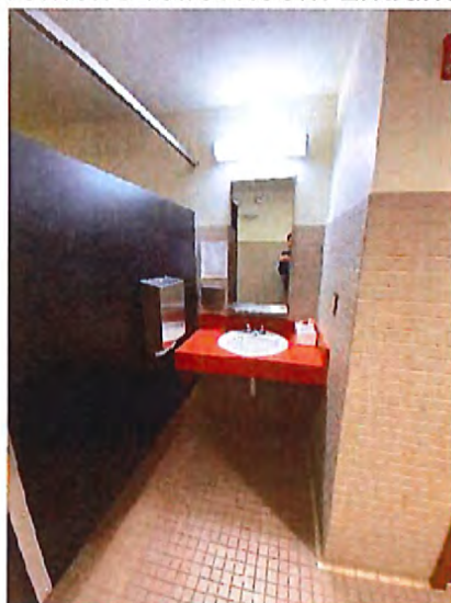
Women's Toilet Room Sink
