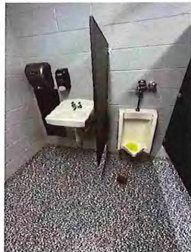
Little League Left Toilet Room Sink
