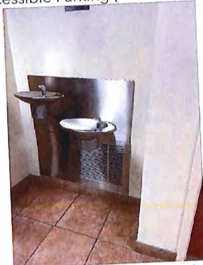
1st Floor Drinking Fountain
