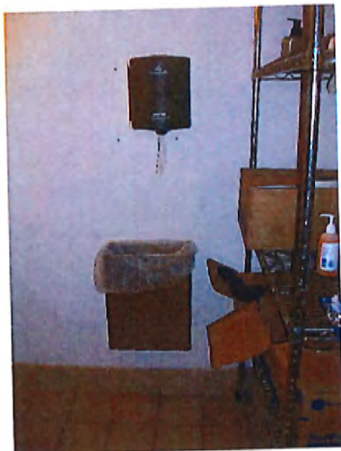
Men's Toilet Room Hand Dryer
