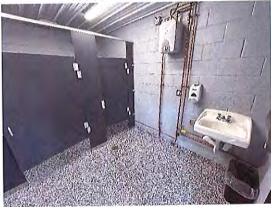
Arts Pavilion Women's Toilet Room Interior
