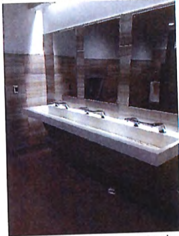
Men's Toilet Room Sinks
