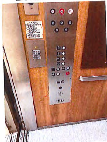
Elevator Control Panel
