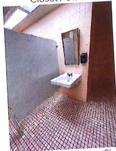
Women's Toilet Room Sink
