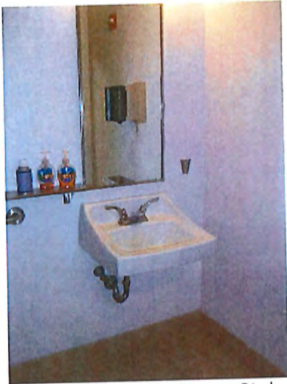
Women's Toilet Room Sink
