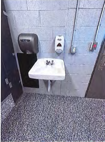
Upper Pavilion - Women's Toilet Room Sink
