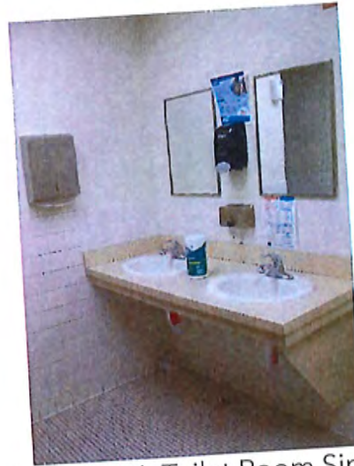
(Left) Men's Toilet Room Sinks
