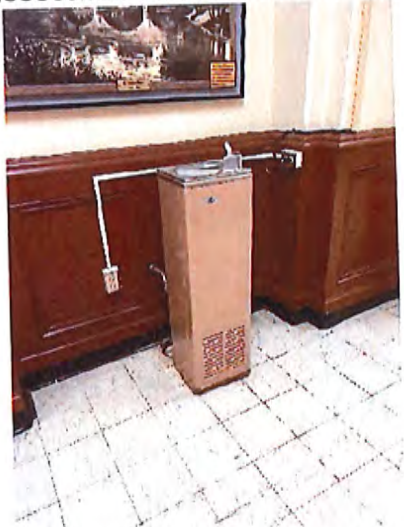
1 st Floor Drinking Fountain
