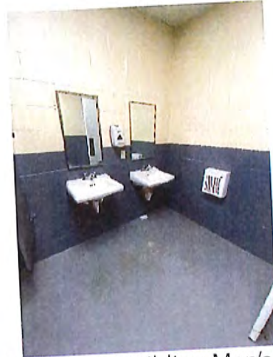
Multi-Purpose Building Men's Toilet Room Sinks
