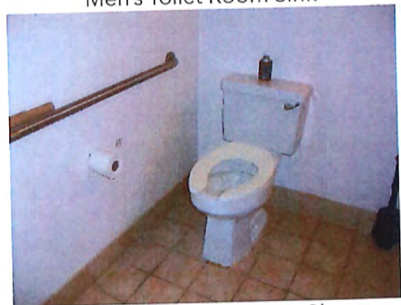
Men's Toilet Room Water Closet
