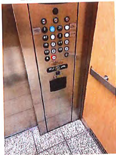
Elevator Control Panel
