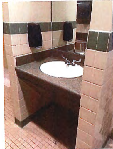
Men's Toilet Room Sink
