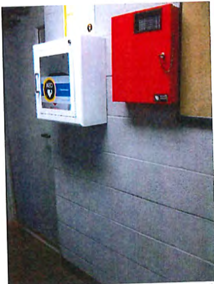
AED / Security Control Panel
