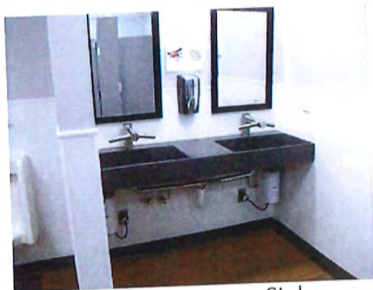
Men's Toilet Room Sinks
