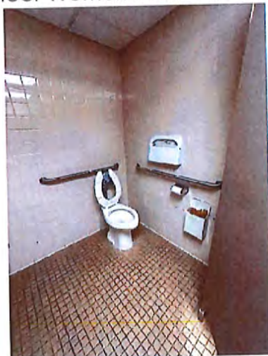
2 nd Floor Women's Toilet Room Accessible Water Closet / Stall
