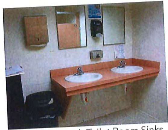
(Right) Women's Toilet Room Sinks
