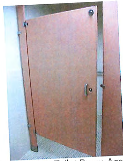
(Right) Women's Toilet Room Accessible Stall Door
