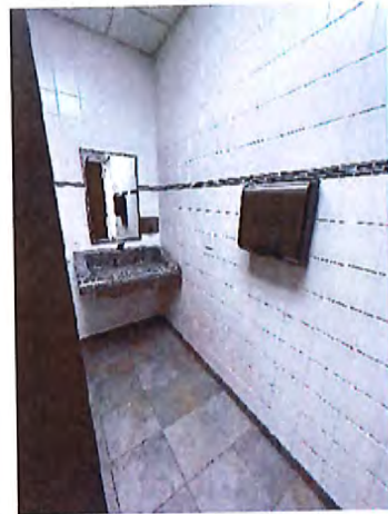
1st Floor Women's Toilet Room Sink
