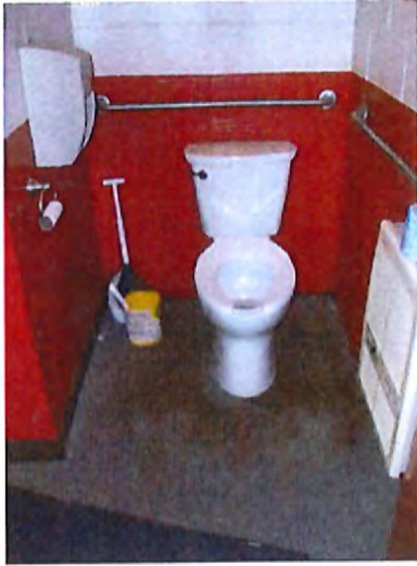
Toilet Room Accessible Water Closet
