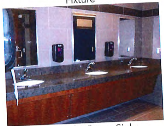
Men's Toilet Room Sinks
