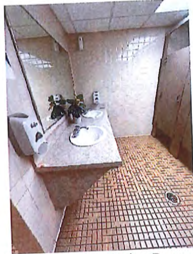
1st Floor Women's Toilet Room Sinks
