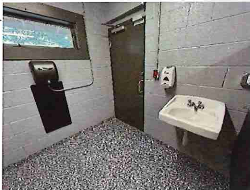
Pavilion #4 Men's Toilet Room Sink
