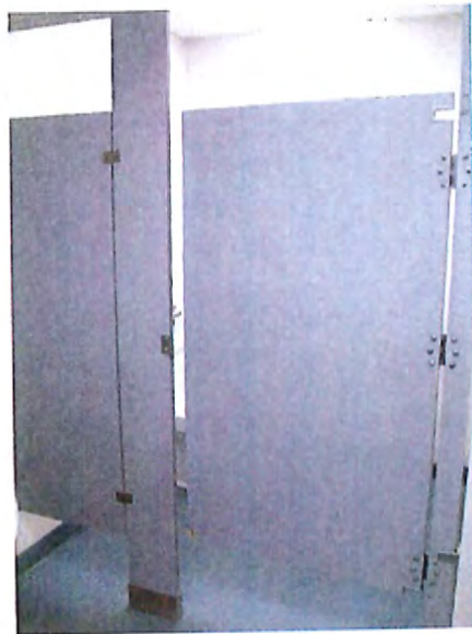
Toilet Room Stall Fixture
