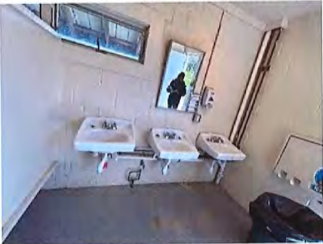
Men's Toilet Room Sinks
