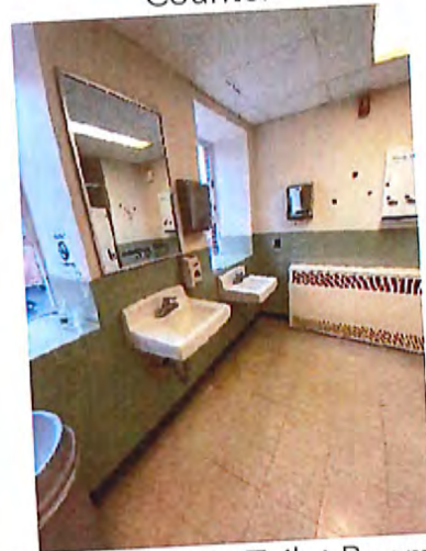
3rd Floor Women's Toilet Room Sinks
