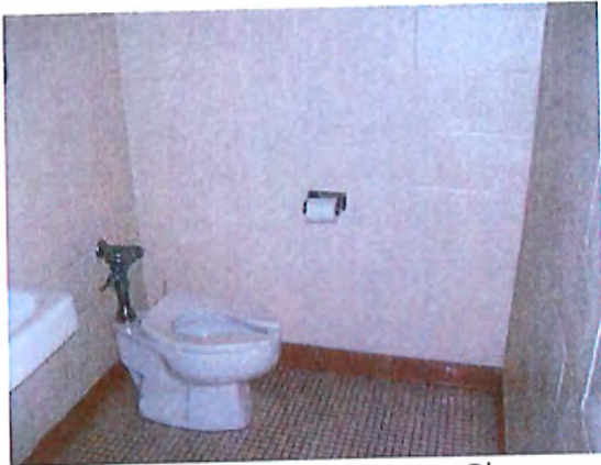
Men's Toilet Room Water Closet
