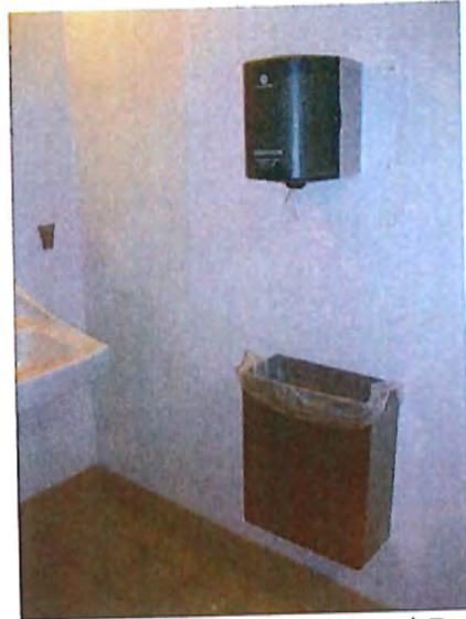
Women's Toilet Room Hand Dryer
