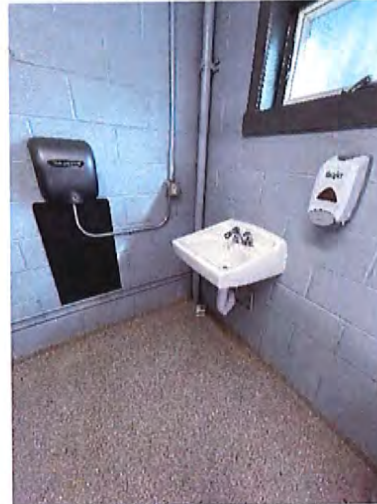
Pavilion Men's Toilet Room Sink
