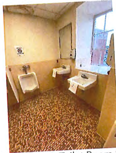
3rd Floor Men's Toilet Room Sinks
