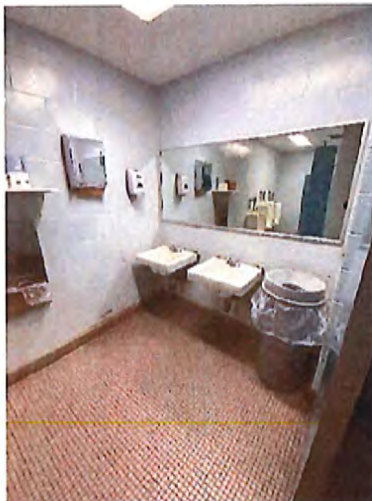
3 rd Floor Men's Toilet Room Sinks
