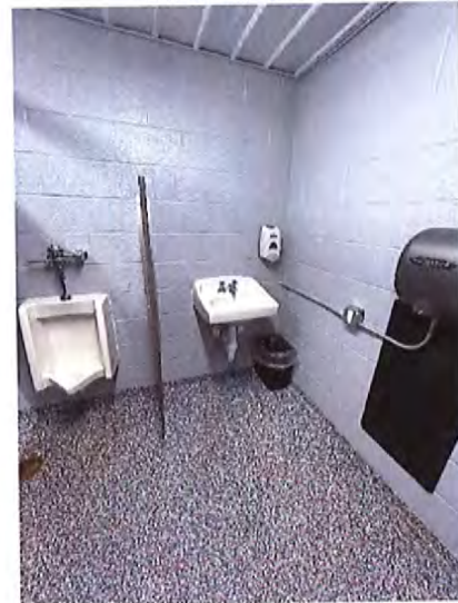
Men's Toilet Room Sink
