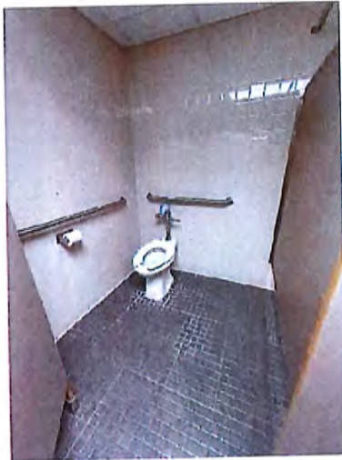
2 nd Floor Men's Toilet Room Accessible Water Closet / Stall
