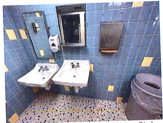
3rd Floor Women's Toilet Room Sinks
