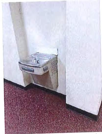
3 rd Floor Drinking Fountain
